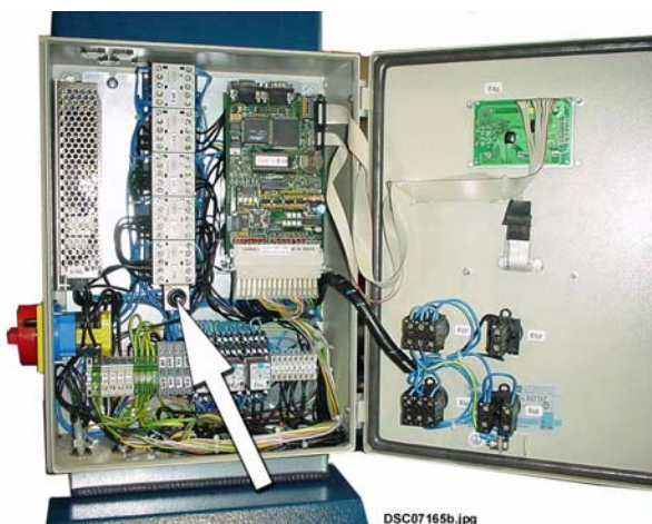
Pic 2: Position of the bypass switch
